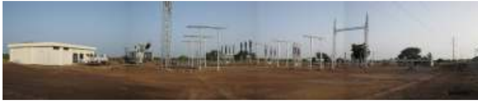
Newly installed Zebila sub-station in Ghana
