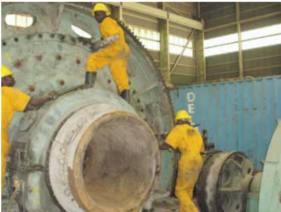
Construction of the 100,000 t/month Kinsenda processing plant involves the relocation and refurbishing of parts of existing concentrator equipment from Musoshi (here) and adding new equipment where required.
