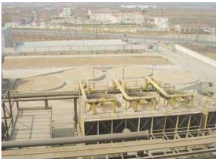
Biogold Bioleaching Facility, Laizhou, Shandong Province, China. View from the top of a Bactech bioleach plant. Note circular cement pads for future expansion (it is about to go to 150,000 ozly).
