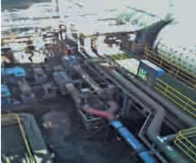
Linatex wear piping
