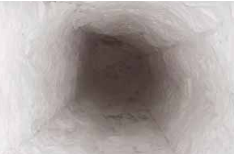
Showing the precision of drilling at the rock face of the raise
