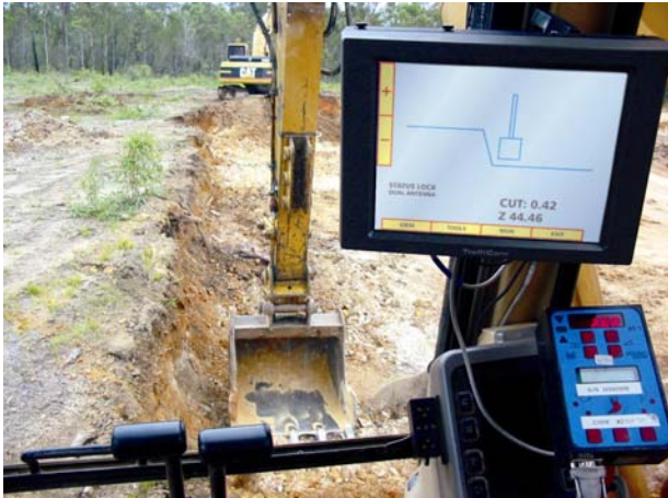
Photo 2 Guidance System being used for excavation of building foundation Excavator guidance from Microfyn, Software from Carlson Software.
