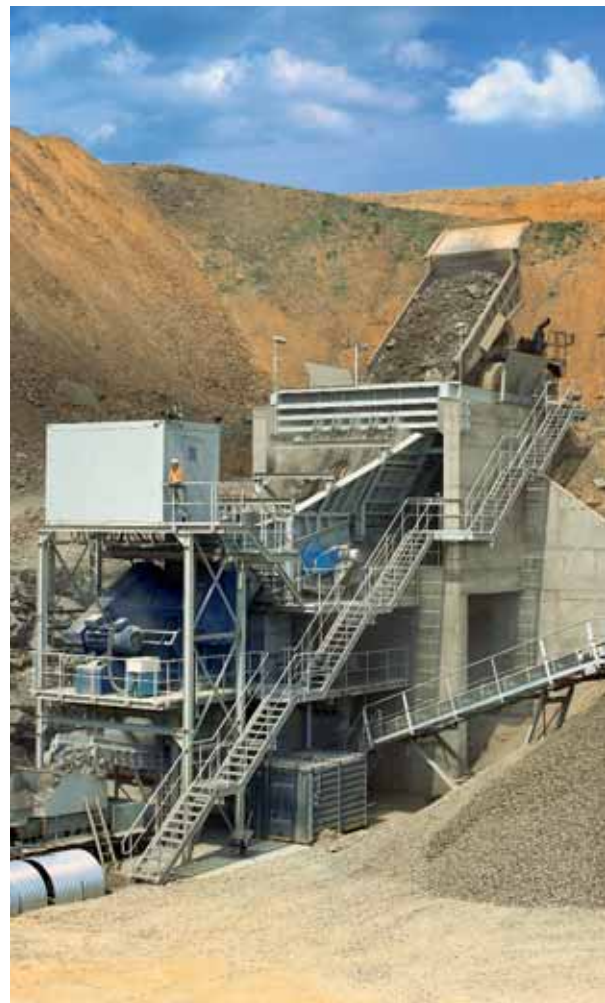
HAVER primary crushing plant with a NIAGARA® scalper DSS 1600 x 4600/3000, Diabas, 500 tons/hr
