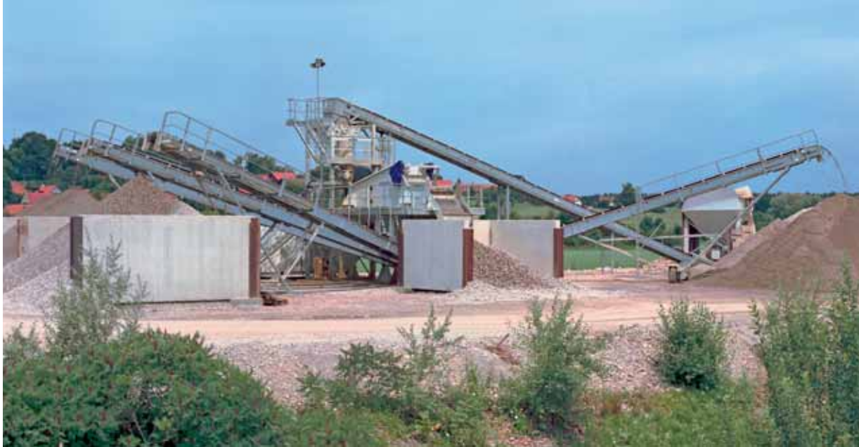
HAYER washing and classifying plant equipped with a HAYER NIAGARA® Flat-Line FL-MD 1200 x 6500/2500 and HAYER Hydro-Clean®, HC 700/80, gravel and sand, 80 tons/hr
